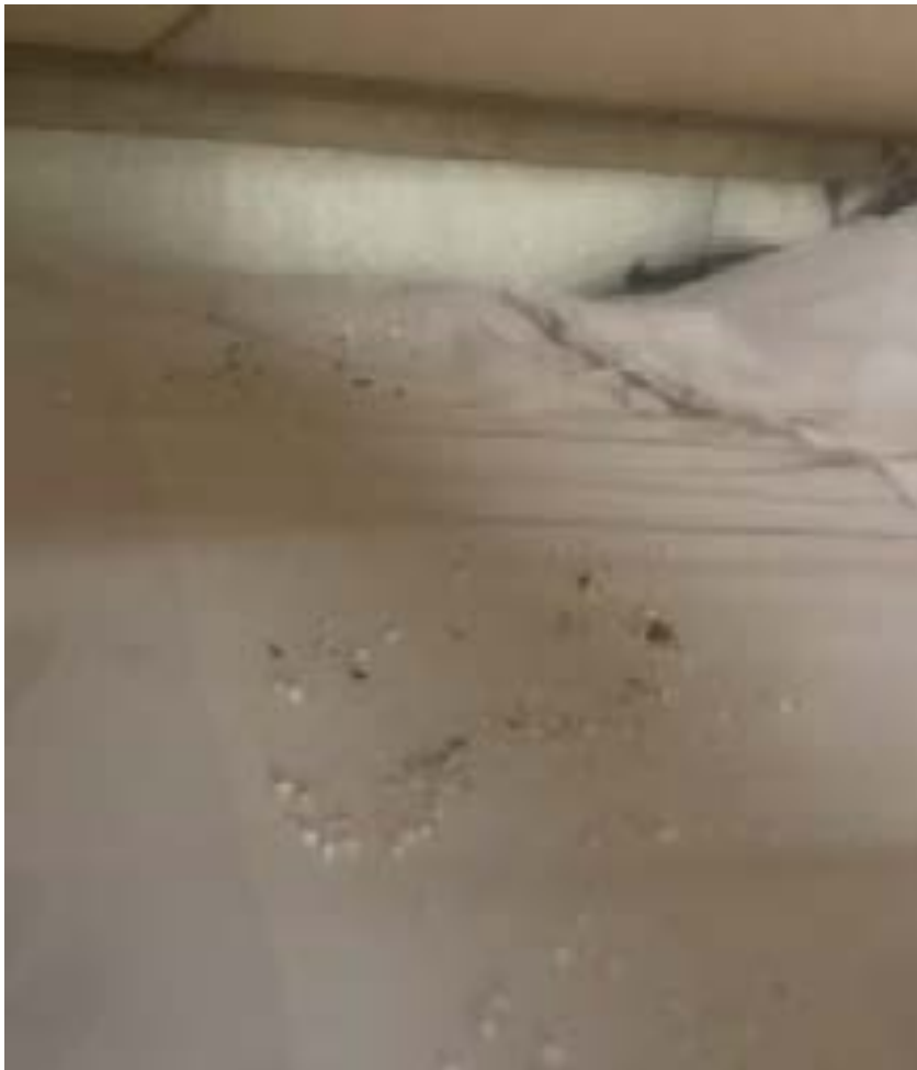
Mouse droppings in roof space
